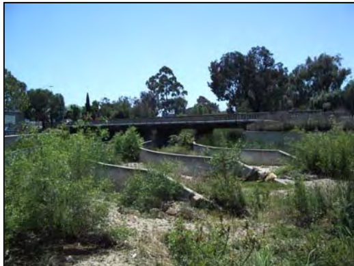
Photo: Figure 5f Date: May 31, 2006 Location: Lower Rose Creek at Mission Bay Drive View: Downstream Flow: Trickle Description: Concrete flow training vanes upstream from Mission Bay Drive.
