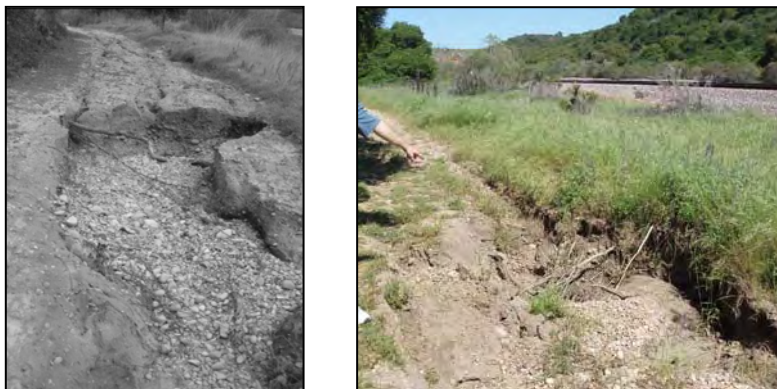
c) Streambed Erosion along Rose Creek
