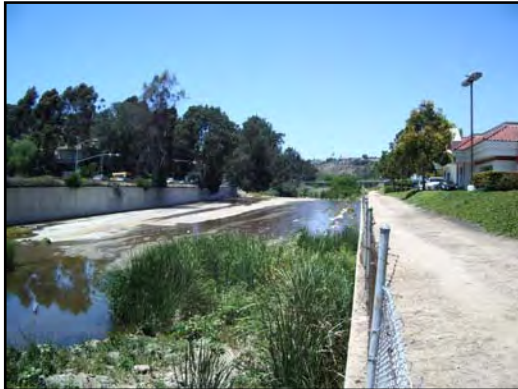
Photo: Figure 5e Date: May 31, 2006 Location: Lower Rose Creek between Interstate 5 and Mission Bay Drive View: Upstream towards Interstate 5 Bridge Flow: Trickle Description: Between Interstate 5 and Mission Bay Drive, the creek is a wide concrete channel with some vegetation.
