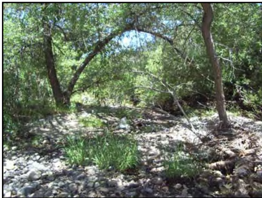
Photo: Figure 4f Date: May 31, 2006 Location: San Clemente Creek west of Genesee View: West, downstream Flow: Trickle Description: Below Genesee Ave, the creek is densely lined with trees. The creek bed is comprised primarily of cobbles.
