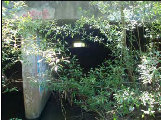
Photo: Figure 3e Date: April 25, 2006 Location: Upper Rose Creek at Genesee Ave View: Downstream Flow: Trickle Description: A triple box culvert diverts flows beneath Genesee Avenue.
