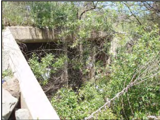
Photo: Figure 4e Date: April 25, 2006 Location: San Clemente Creek at Convoy Street View: Upstream Flow: Trickle Description: The culvert at Convoy Street near the landfill. The photo also shows the vegetation increasing farther downstream.
