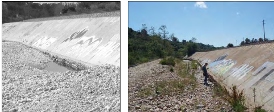
b) Streambed Erosion below Concrete Bank along Rose Creek near Interstate 805
